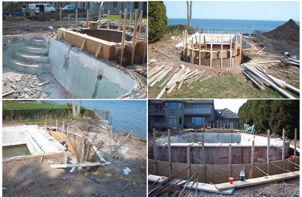
Various stages of restoration: In order to succeed, in terms of what the client had in mind, Oasis had to perform a complete overhaul of the existing, four-decade old concrete swimming pool that was in extremely poor condition. To bring the swimming pool back to life, the concrete structure was sandblasted to clean the surface, while new coping, tile, marbelite, staircases, skimmer and circulation lines were added. The facelift also included incorporating an elevated gunite hot tub, a spill over edge and dual corner staircases.
